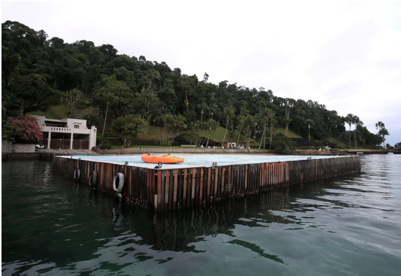
Figure 10: Helipad on the Morcego beach: ostentation invades the ocean, photo by Júlio Cezar Guimaraes, 2017. 69
